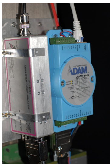
Figure 6. High Voltage (HV)
